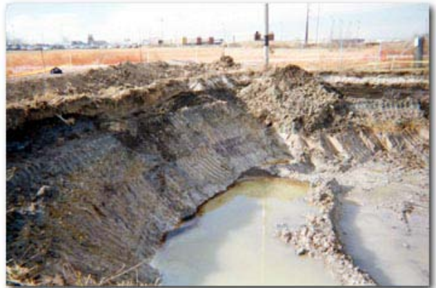
Free product oozing into open excavation at Moss-American site in 1995-1997. Photo from EPA Region 5 website.
