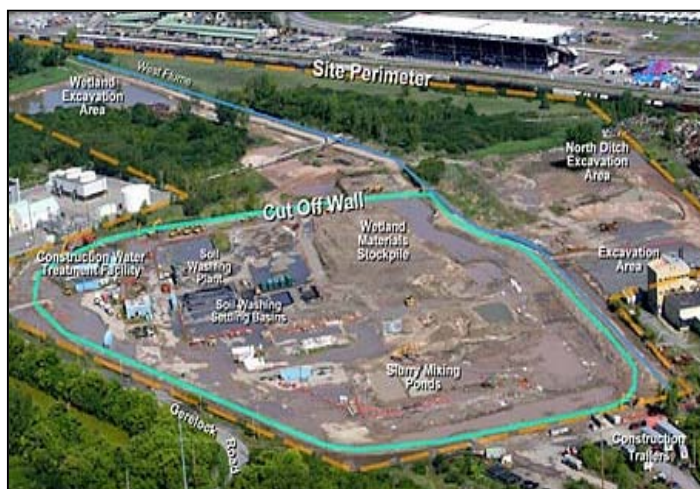
Onondaga Lake Bridge Street subsite (OU 5) with mercury remediation system. Photo from www.onondagalake.org
